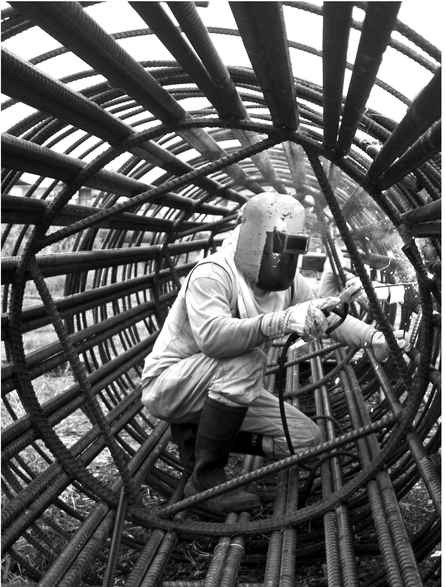
Man working inside a large reinforced steel tube. Philippines. Photo: Nonie Reyes / World Bank
